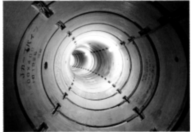
図17 R = 15m超急曲線推進完了後の洞道 Fig. 17 Inside of jacking pipe route of 15m radius after completion of thrusting work
