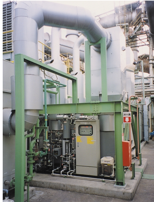
図6 ボイラと排ガス処理装置 Fig. 6 Outline of boiler and exhaust gas processor
