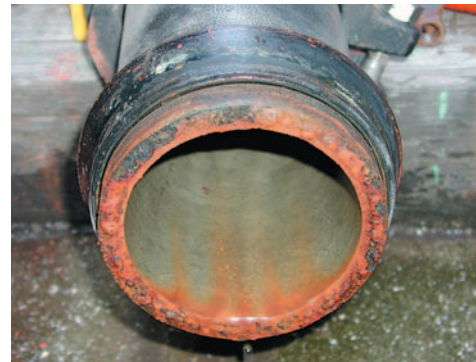
図12 非防食部(3年経過後) Fig. 12 Non-corrosion prevention part of cutting section (Passes in three years)
