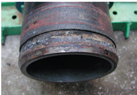
図11 防食部(3年経過後) Fig. 11 Corrosion prevention part of cutting section (Passes in three years)
