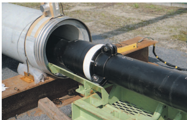
図14 直線管路での施工試験 (NS形) Fig. 14 Construction test into straight line casing pipeline (NS-type joint)
