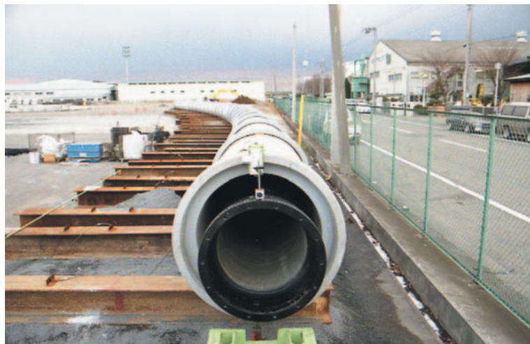
図13 S字カーブ管路での施工試験 (S形) Fig. 13 Construction test into S-curve casing pipeline (S-type joint)
