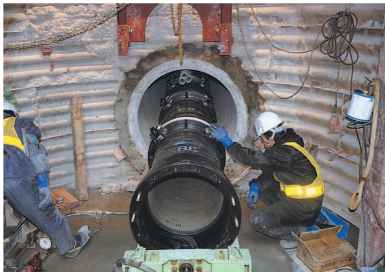
図18 発進立坑における施工状況 Fig. 18 situation of the construction in launching vertical shaft
