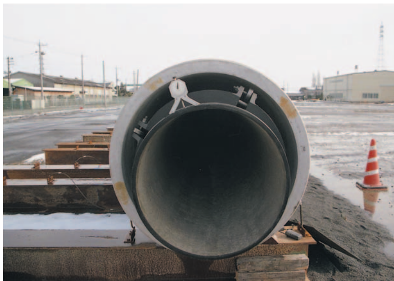
図15 Sカーブ管路到達側のローリング角度測定 Fig.15 Measurement of rolling angle at the end of S-curve casing pipeline
