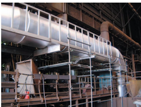
図6 熱風ダクト更新工事 Fig. 6 Renewal construction of the duct for hot blast
