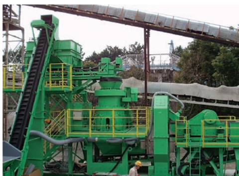
図6 設備全景 Fig.6 Whole view of equipments
